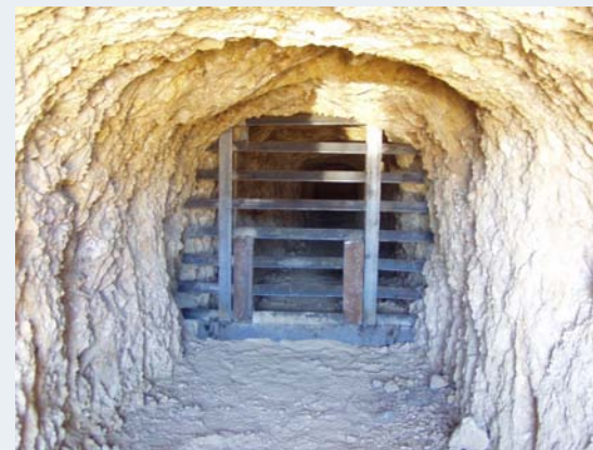
This bat gateway installed on a mine in Nevada to protect the largest known maternity colony of Pallid bats in Nevada. These gates are installed to protect hibernating bats as well as colonies of females giving birth. The first few weeks following the birth of pups is a very vulnerable time. Photo by Jason Williams.
